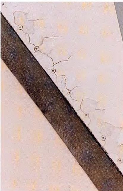
Paint system is too thick
